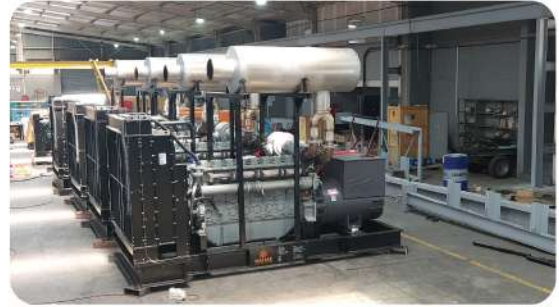
1000kVA Open Set
